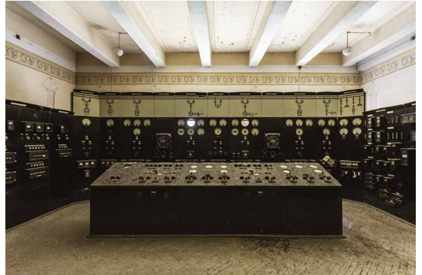
Control room of a hydropower plant near the Chechen border. We had to walk more than 15 kilometres to get here. Surprisingly, it was a rather pleasant hike.
