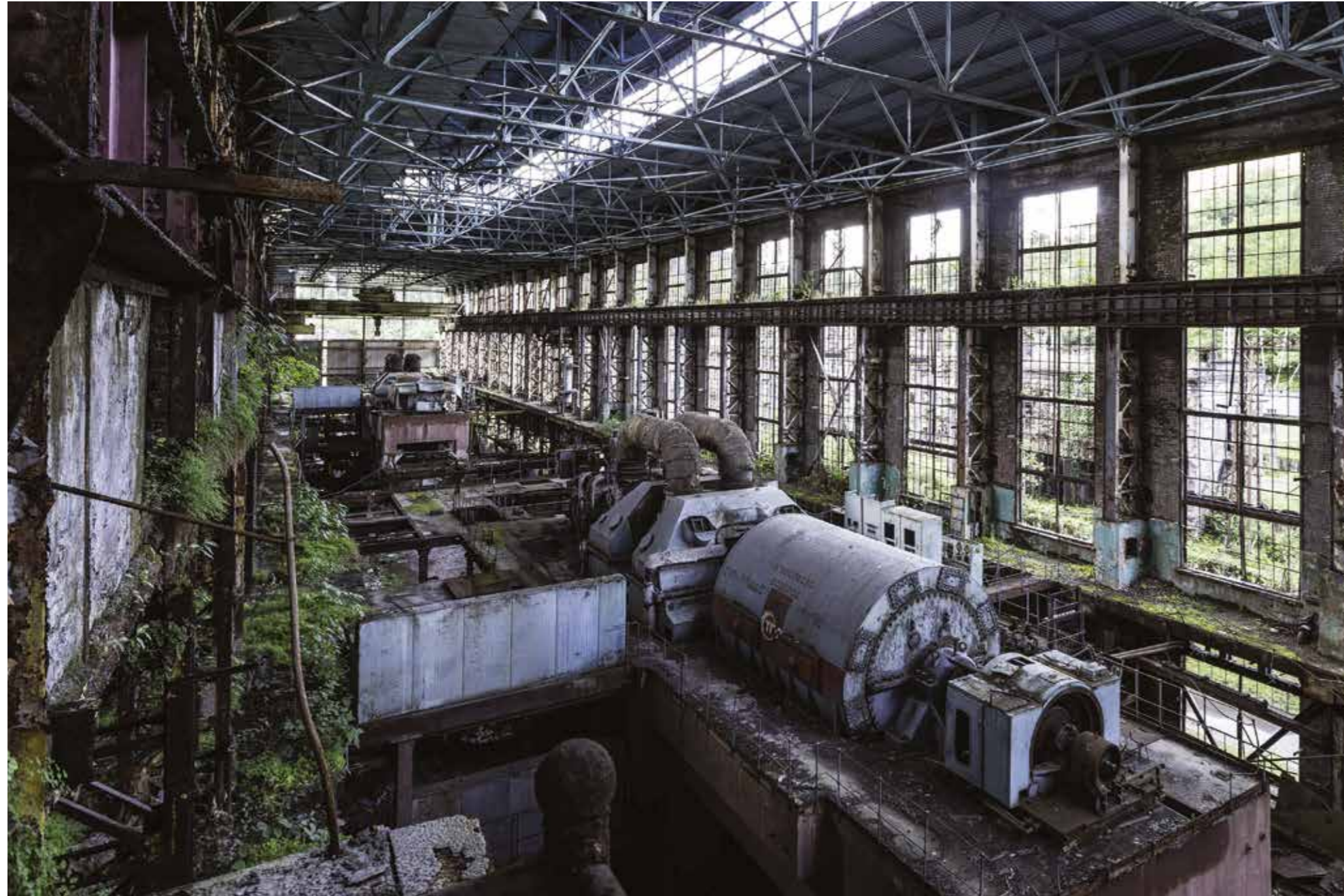
Large turbine room in Tkvarcheli power station.
