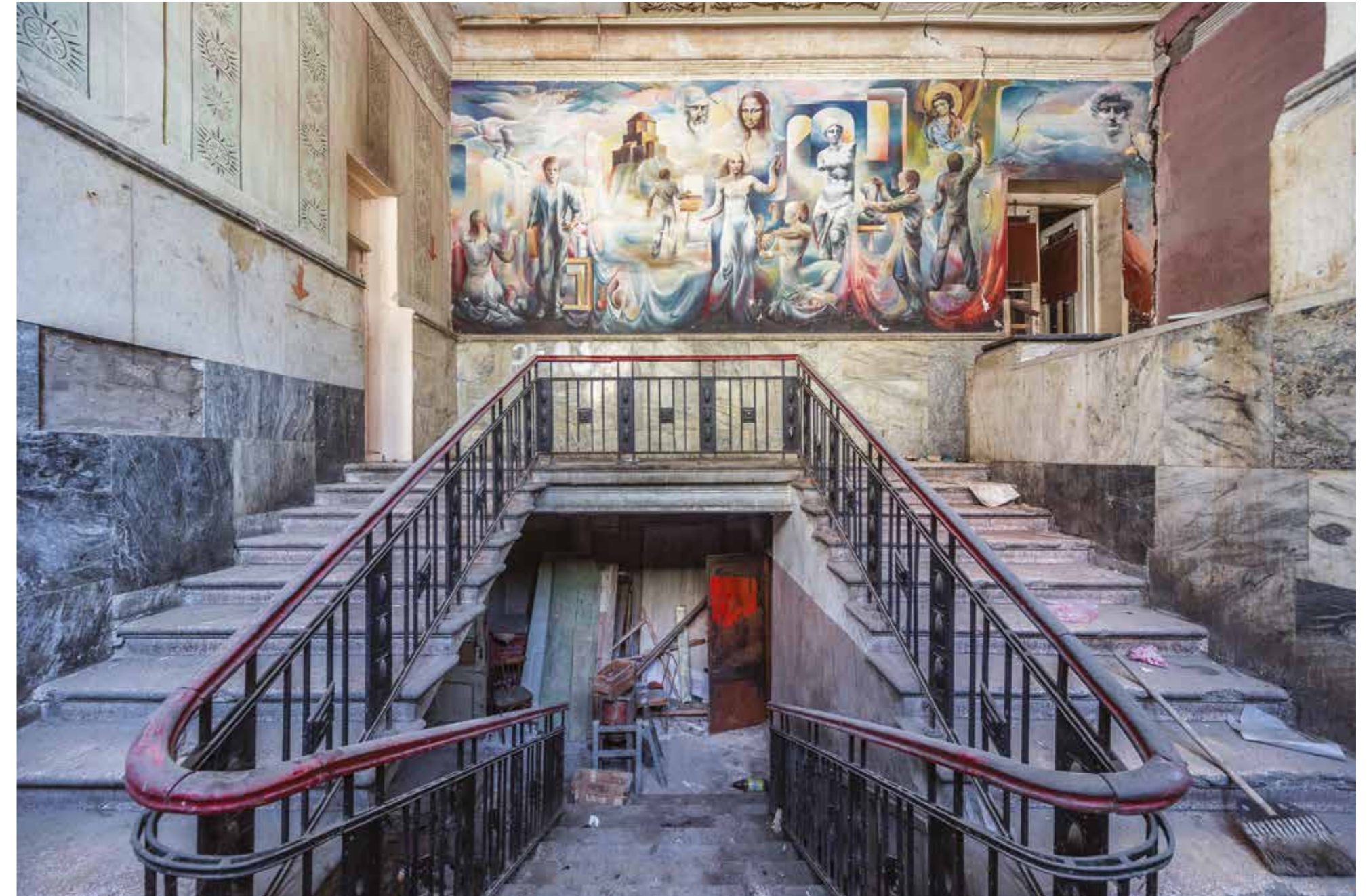
Abandoned School of Art in the centre of Tbilisi. The cracks in the wall on the right were caused by the 7.2-magnitude earthquake that severely damaged the capital in 1991.
